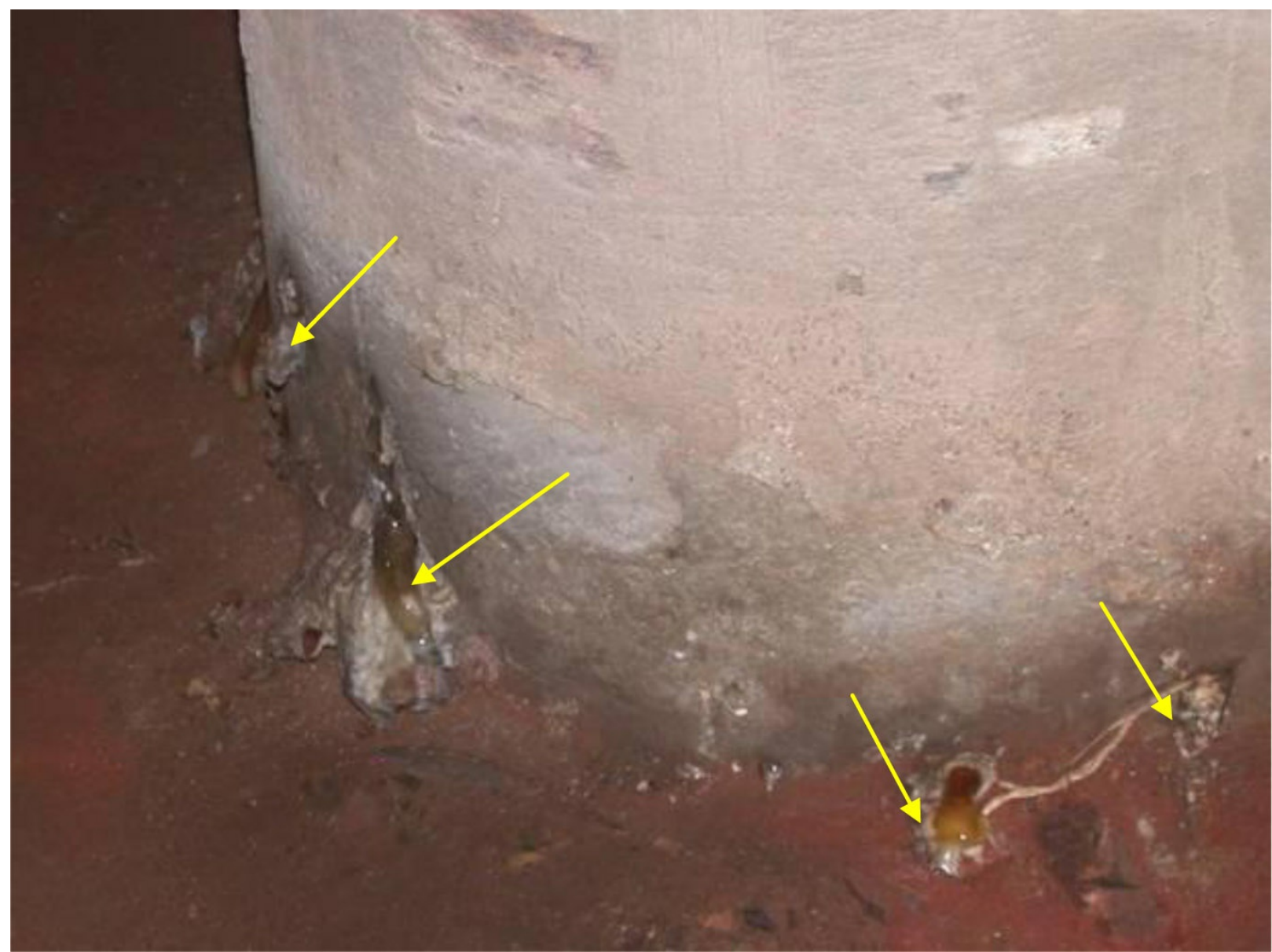
Figure 1: ASR Gel Exudations at Base of a Shed 1 Pile (arrowed)
