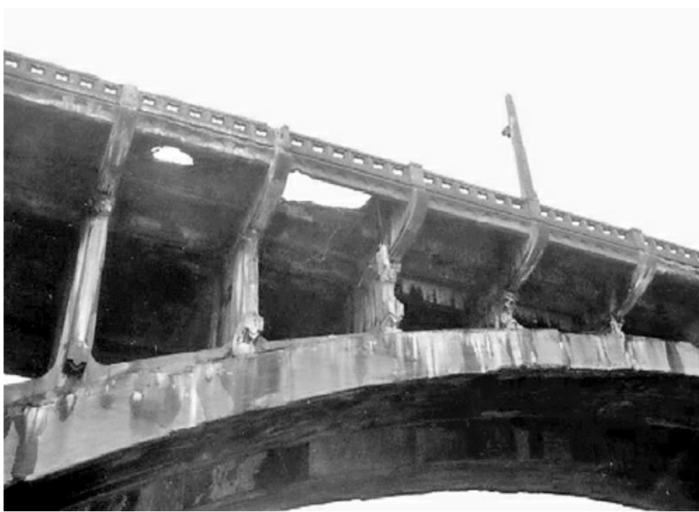
FIGURE 4 Corrosion-Induced Damage on Bridge Deck
