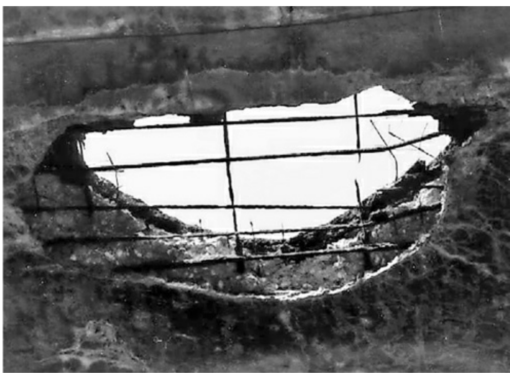
FIGURE 1 Loss of Cross-Section of Reinforcement as a Result of Corrosion
