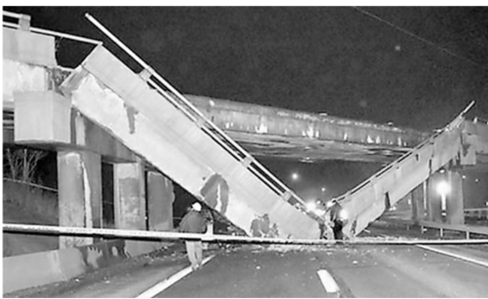
FIGURE 3 Collapse of I-70 Overpass as a Result of Prestressing Cable Corrosion
